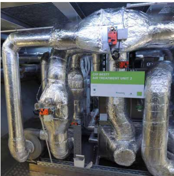
ATU – Air Treatment Unit, high accuracy air conditioning system for flight condition simulations
